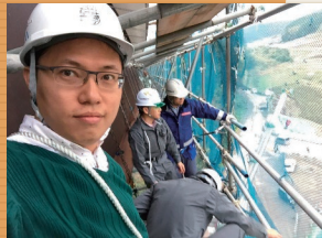
I really enjoyed visiting the site of road rehabilitation because I was able to improve my knowledge and it was very helpful in my work and research.
